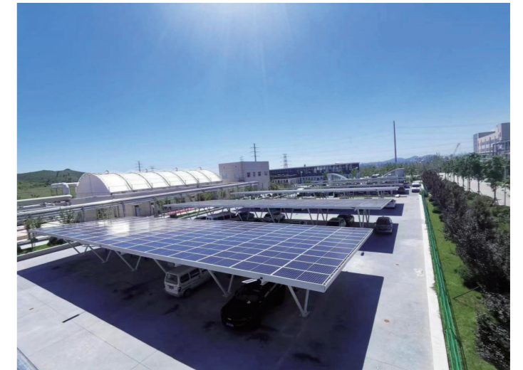
Photovoltaic power generation equipment
