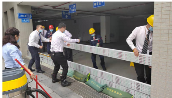
Waterproof baffles and sandbags were laid at the flood entrance on site
