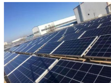
河北长安光伏电站 Hebei Changan Photovoltaic Power Plant
