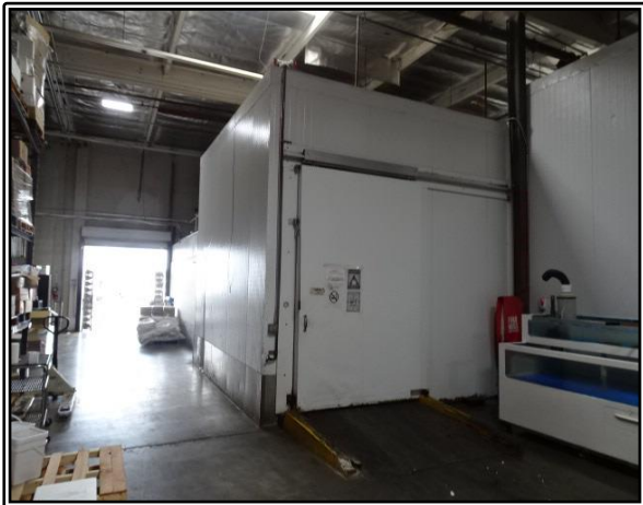
Unit 1146 cold storage box.
