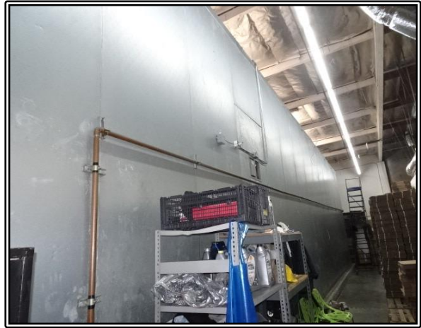
Unit 1150 cold storage box.
