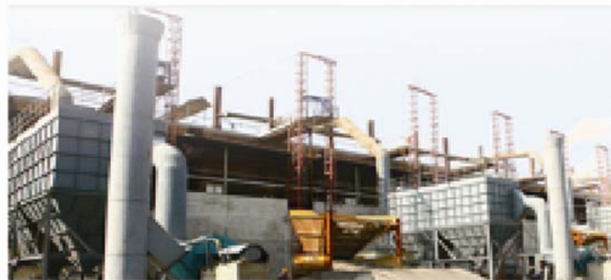
三岩厂区 (Processing Plant of Sanyan)
