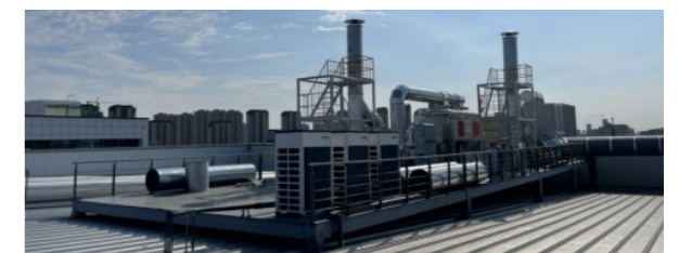
Equipment for Catalytic Combustion in Emissions Control
