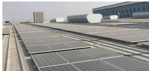
Photovoltaic Panels at the Haier Biomedical Industrial Park
