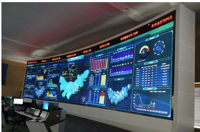
Figure 6: Commanding Center for Electric Power Dispatch
